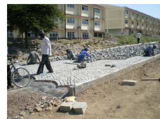
A pedestrian walking on cobblestone paved walkway at Adama UCBP site.
